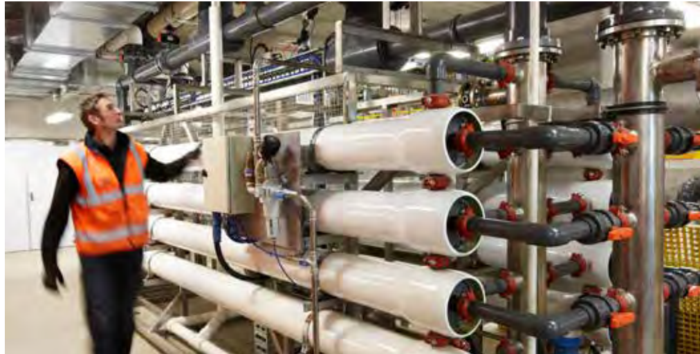
Yarra Park Recycled Water Treatment Facility
