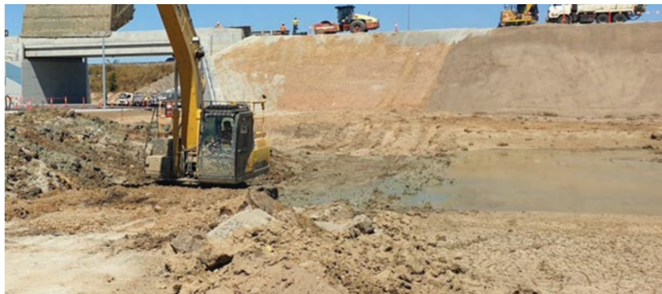
Application of Slurry Thick with Excavator July 2022 – Image Courtesy of Georgiou Group
